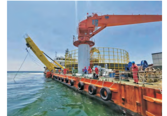
三峡新能源阳西沙扒一~五期海上风电项目/220kV Three Gorges Yangxi Shapa Offshore Wind Power Project
