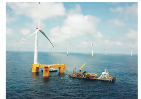
三峡广东浮式海上风电项目动态缆 Dynamic Cable of the CTG Guangdong Floating offshore Wind Power Project
