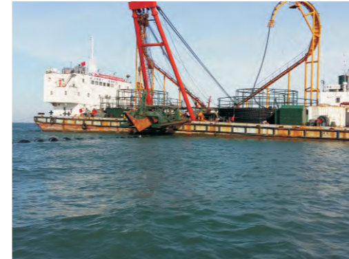
龙源福建莆田南日岛海上风电场项目/220kV Longyuan Fujian Putian Nanri Island Offshore Wind Farm Project
