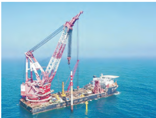
广东华电阳江青洲三500MW海上风电项目/35kV Guangdong Huadian Qingzhou Three 500MW Offshore Wind Farm Project
