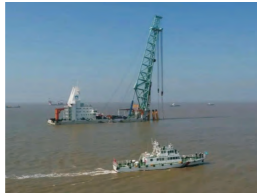
浙江华电台州玉环一期300MW海上风电项目/66kV Zhejiang Huadian Station Yuhuan Phase I 300MW Offshore Wind Power Project
