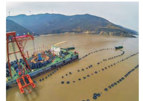
舟山多端柔性直流输电示范工程/±200kV Zhoushan Multi-terminal DC Flexible Transmission Demonstration Project
